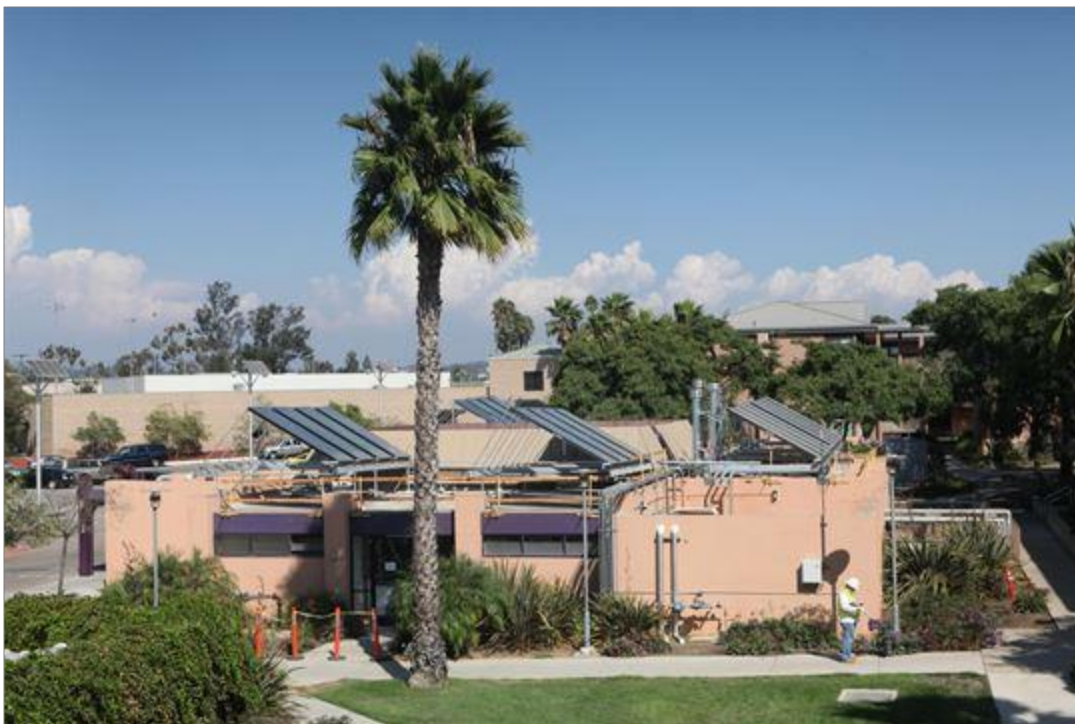
Solar panels on MCAS Miramar buildings
